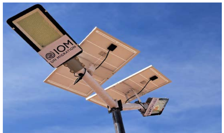
Solar lights installed to enhance protection in IDP gathering sites in Wad Medani, Aj Jazirah state. © IOM SUDAN 2023
