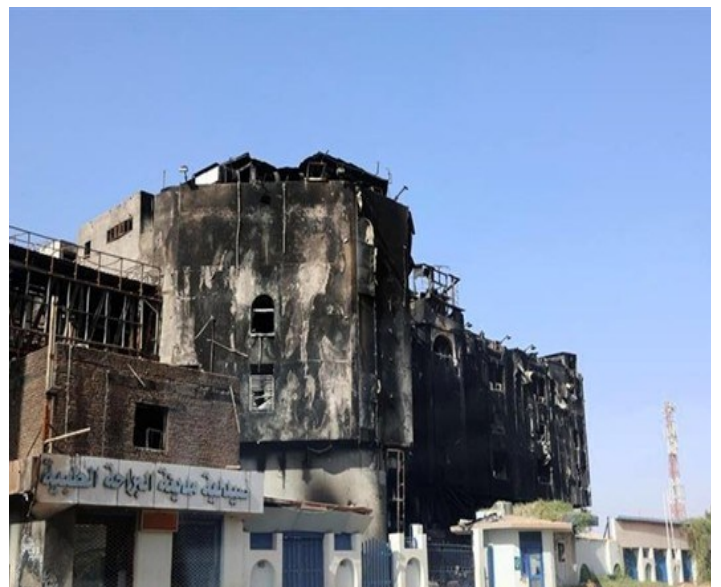
DESTROYED HOSPITAL IN BAHRI, KHARTOUM - APRIL 2025 IOM
